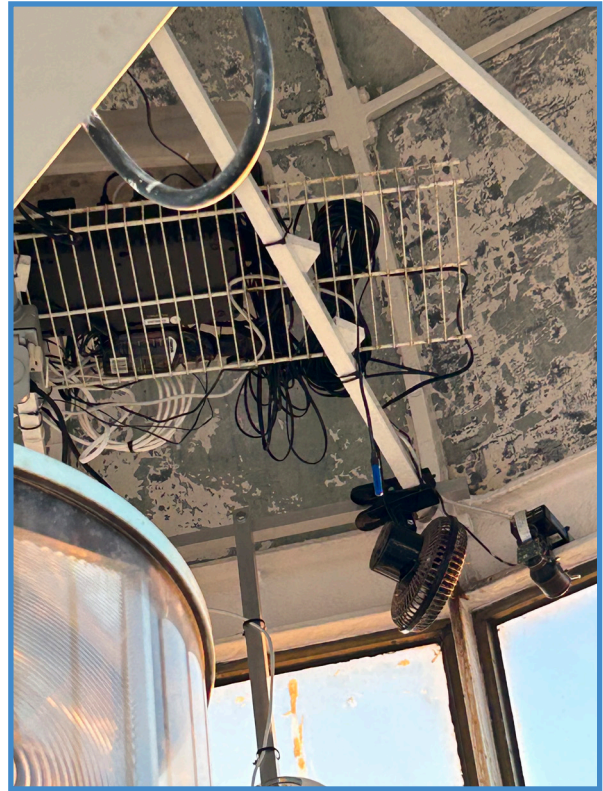
IT Equipment Installation - notice Room Alert environment monitoring Digital Temperature & Humidity Sensor
